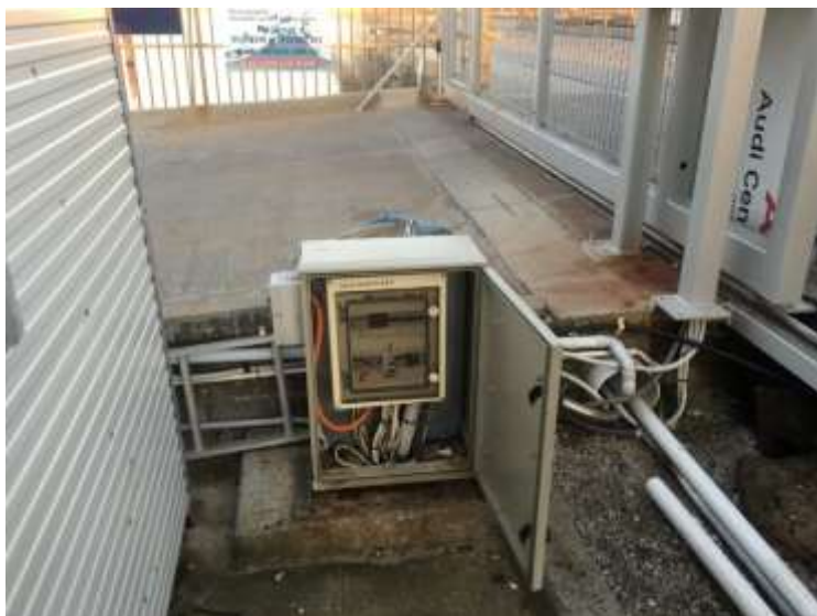
Electrical Shut-Off – Brighton Pier
